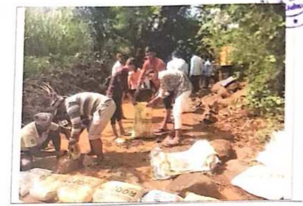
Students of National service scheme, Villagers and Dr. M.K. Kambik, Coordinator National service scheme, while building an embankment of forestry method on mouje malwadi stream.
