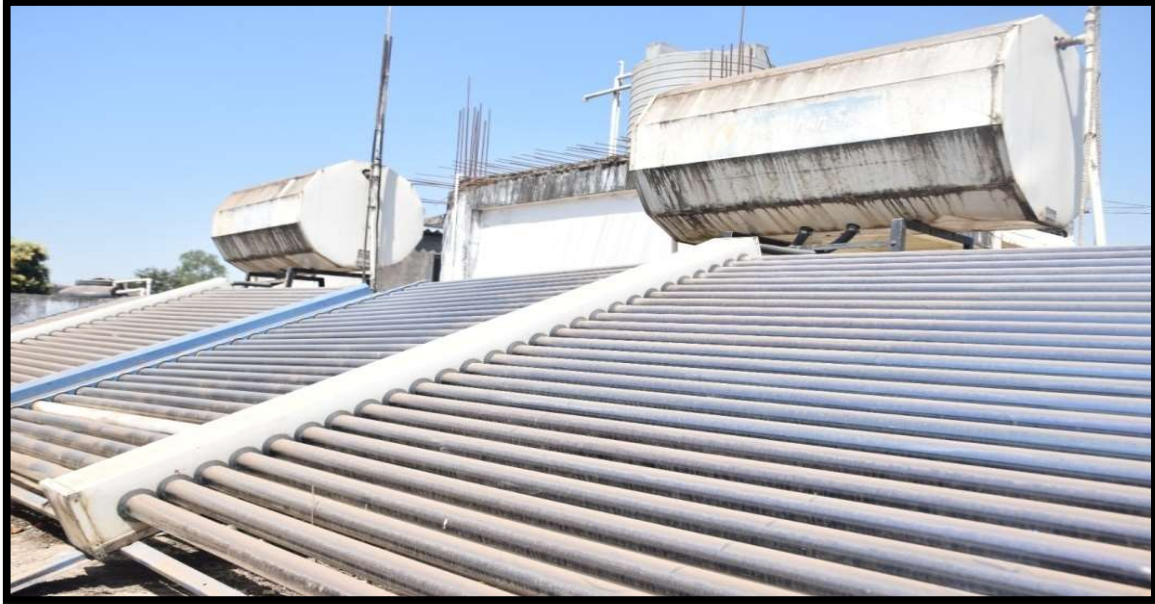
Solar system installed on top of boy's hostel
